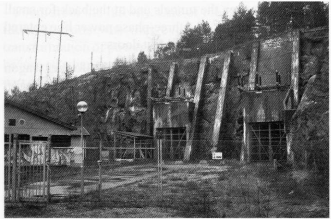
The converter station at Nyköping is still in use, seen here in March 2008. Photo by Lars Hansson
